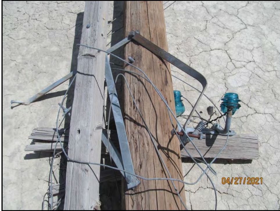
Log 1, Image 20, 26Wa12841, H-3 Detail of hardware components (Plan) Praana II Washoe BESS/PSES Site Project, UTM Zone 11, 245836 E/ 4449440 N
