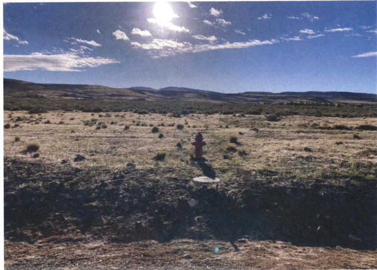
View east from Cielo Vista Drive with water main and fire hydrant.
