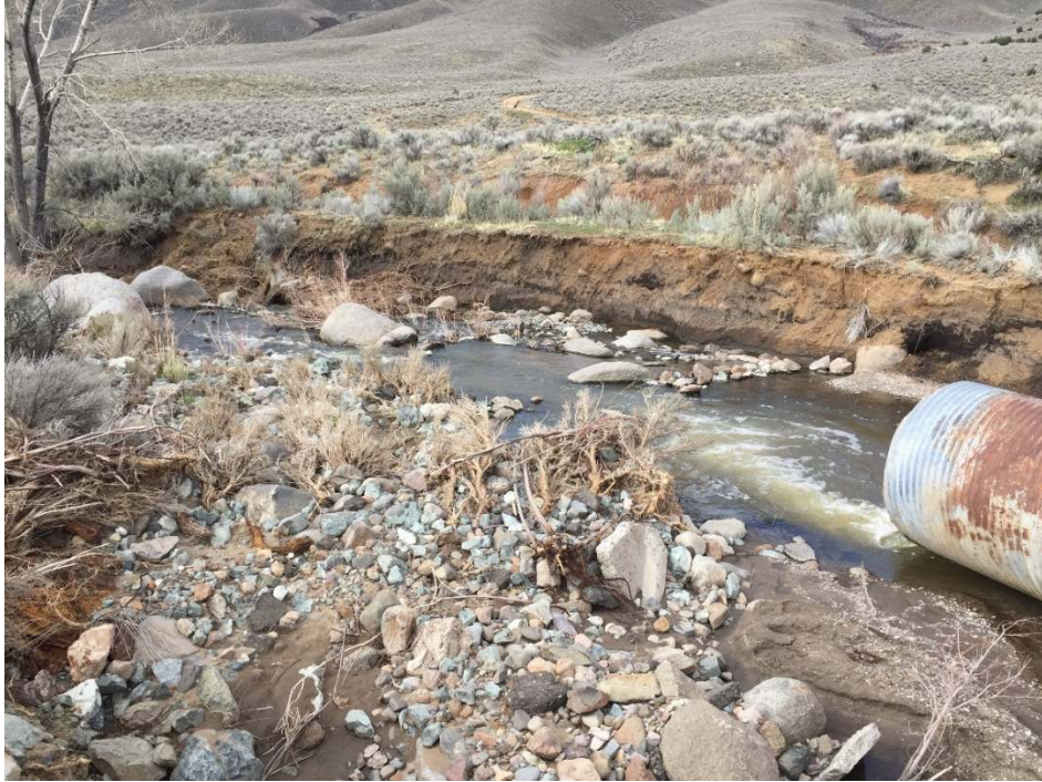
Downstream damage to creek from Washed out Culvert
